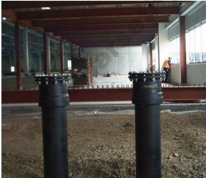
Photo 8: Prepared connection to the sprinkler sub-central room
