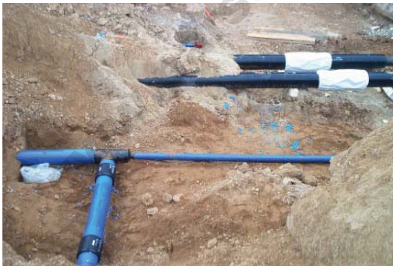
Photo 2: Agruair compressed air pipe and fire main (background)
