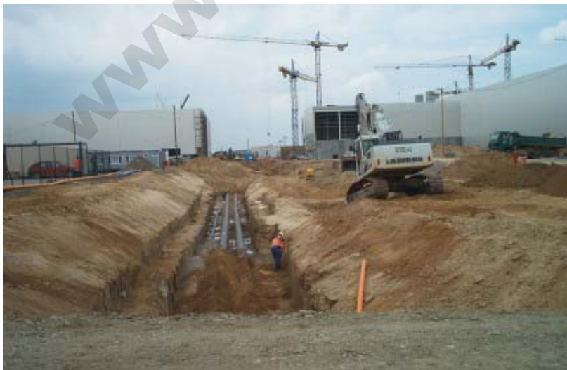
Photo 6: Parallel connecting pipeline to a sprinkler sub-central room
