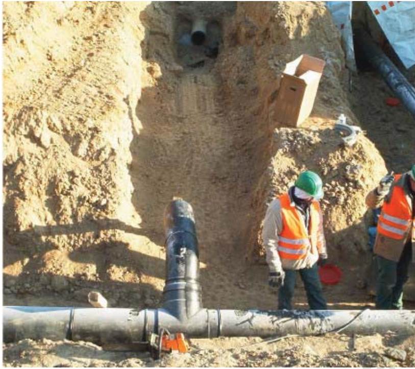
Photo 7: Branch from the main pipeline (DN 300) to the sprinkler sub-central room (DN 250)
